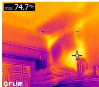
Missing Insulation – Summer Day E6 with MSX
