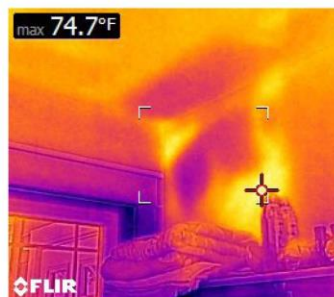
Missing Insulation – Summer Day E6 with MSX
